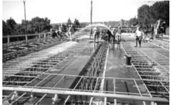
Fig. 2.2—GFRP bars installed during the construction of the Crowchild Bridge deck in Calgary, Alberta, Canada, in 1997.
