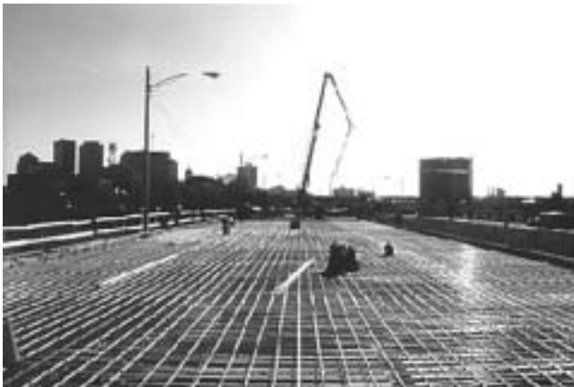
Fig. 2.5—GFRP bars used in the redecking of Dayton, Ohio's Salem Avenue Bridge in 1999.
